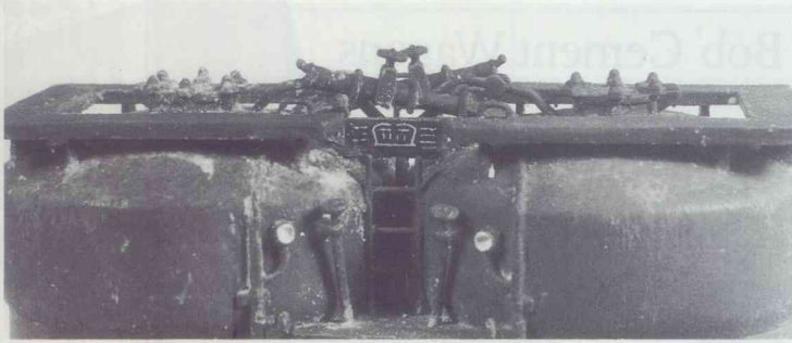
The pipework on the Prestwin, larded with muck and dust — interestingly complex, yet relatively quick and easy to do.
